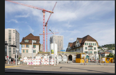
2023 Construction site of the tram depot for coop- erative housing (Wenger Timon)
