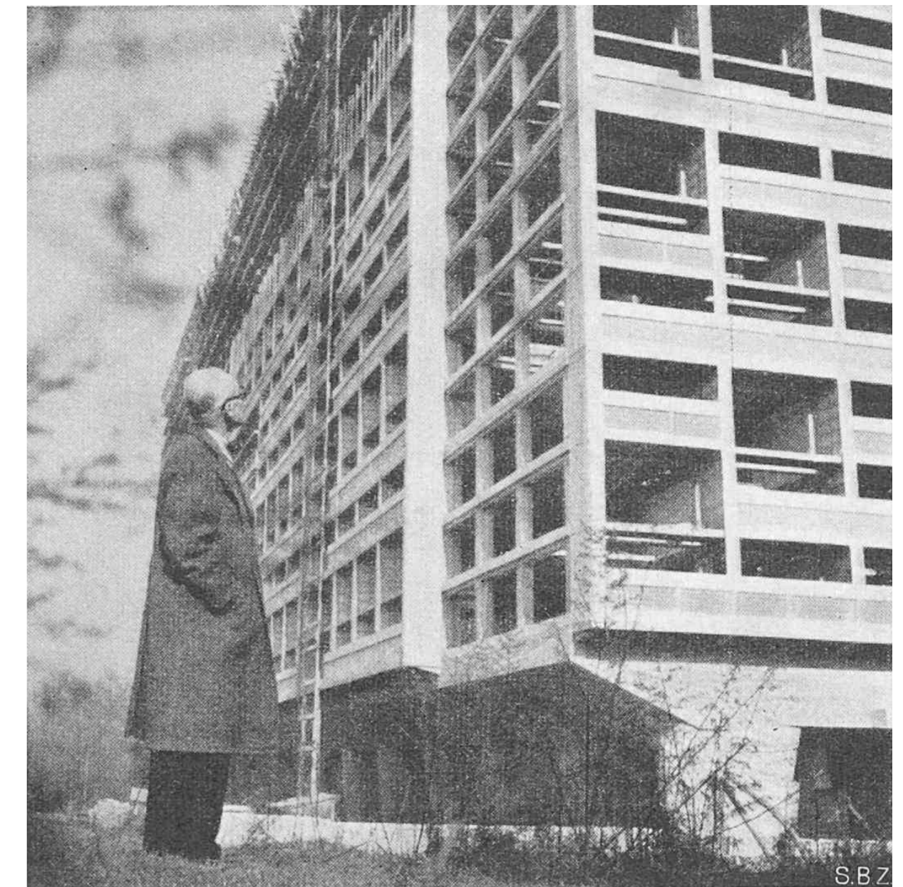
Le Corbusier in front of the carcass of the Unité d'Habitation. A Model that has spread as a model even before it was built. Picture from around 1949, published in 1950 12
